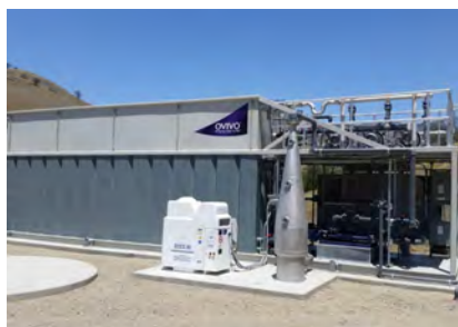
Ovivo's water treatment plant in Canton is playing host to a pilot project using UA algae technology
